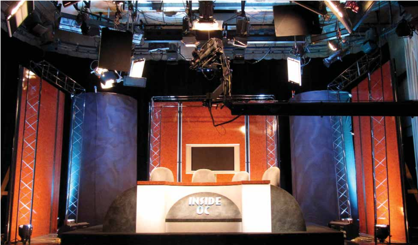
ParaBeam® 410 DMX, lighting public TV broadcast studio
